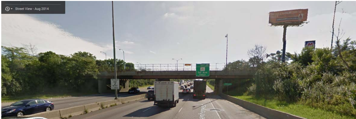
View of slightly depressed I-290 roadway profile and use of concrete barriers at 17 th Avenue.
